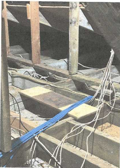
Compromised roof trusses
