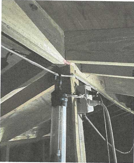
Electrical-not to code (3)
