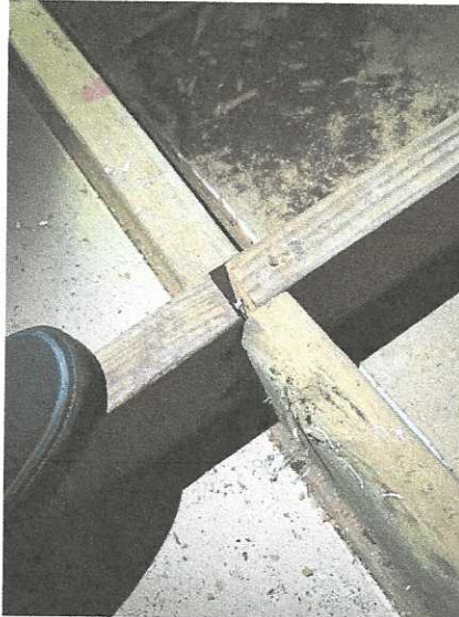
Missing structural hardware
