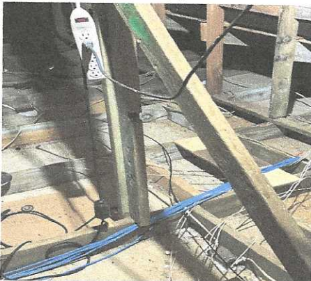
Electrical-not to code (5)
