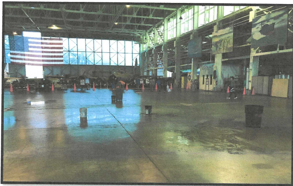
Current condition of Hangar 79's roof allows rain water to leak through, creating safety issues for staff and visitors. Hangar 79 is currently partially closed to the public, with majority of the aircraft removed.
